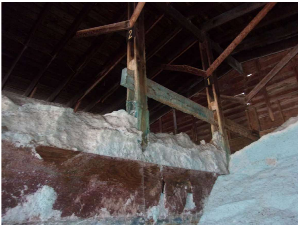
Photograph S-28: Typical Broken / Failed Knee-Bracing
