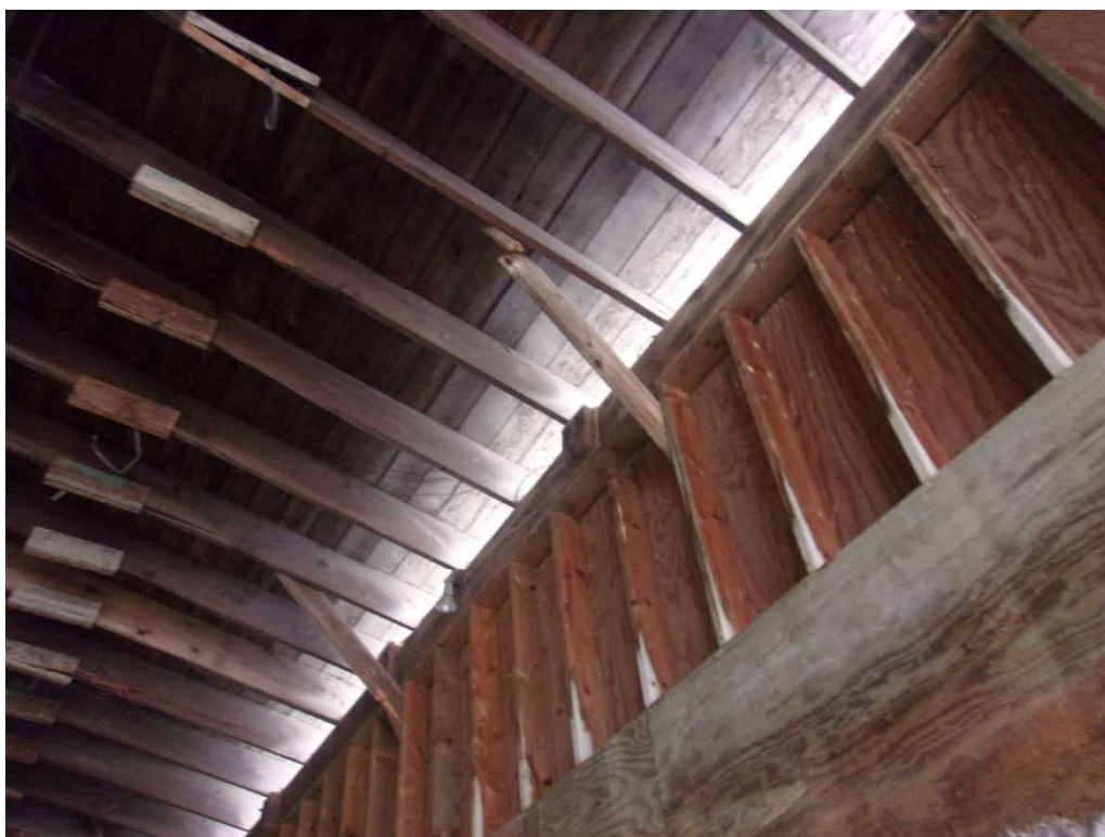
Photograph S-29: Typical Broken / Failed Knee-Bracing
