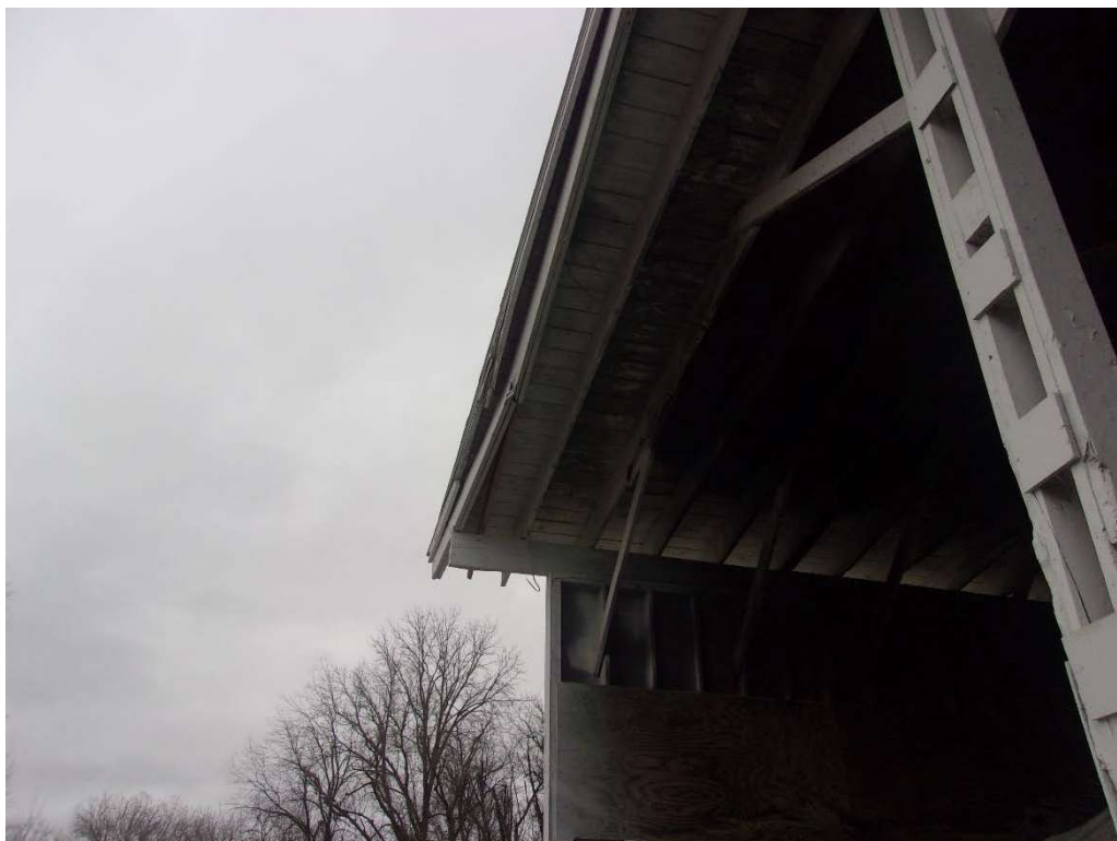
Photograph S-27: Cracked / Broken Rafters at Gable End (Open End)
