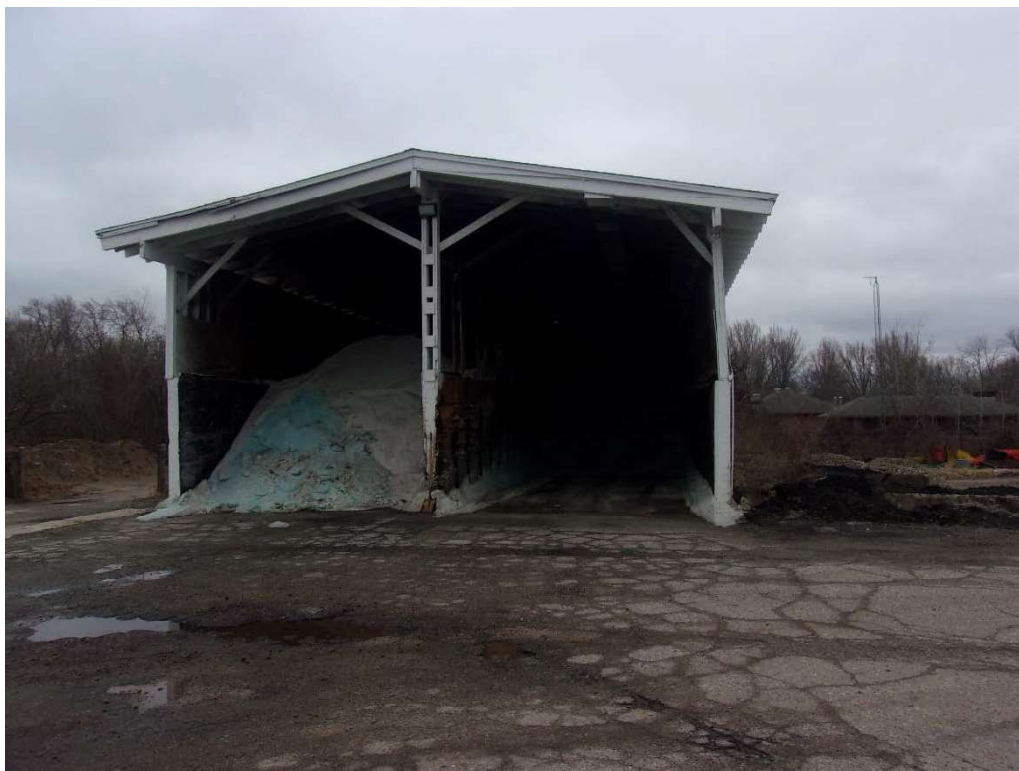
Photograph S-23: West Concrete Wall slightly Out-of-Plumb
