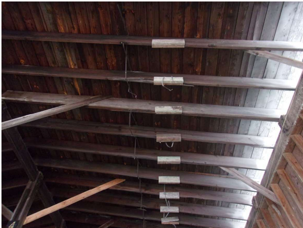
Photograph S-26: Typical Cracked / Split Roof Rafters
