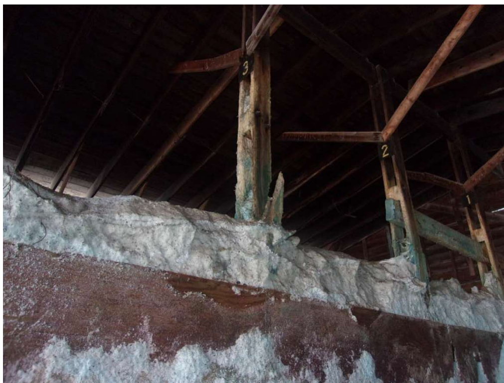
Photograph S-24: Center Column Cracked / Failed Above Barrier Wall
